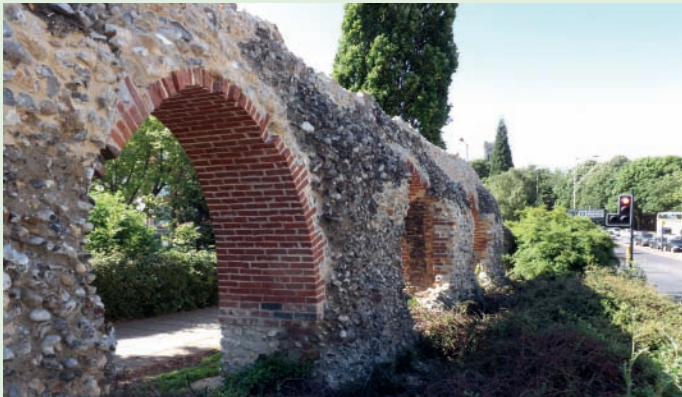
View of the repaired section of wall at Barn Road 2015. Photograph: Vicky Manthorpe.
